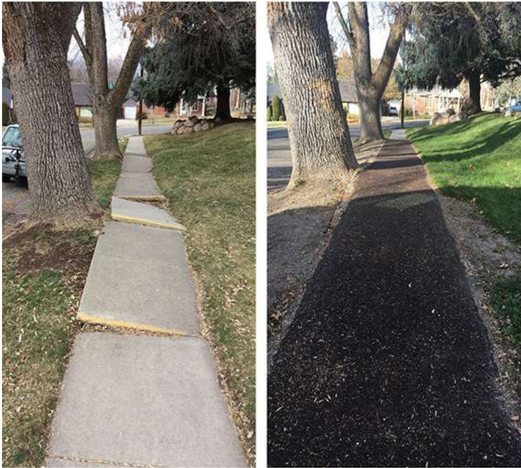
Damaged sidewalk (left) that was replaced with permeable pavement (right) in 2018 in Ogden, Utah.
